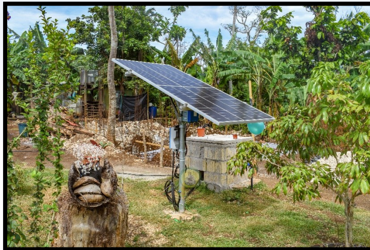
A solar water pumping system in
