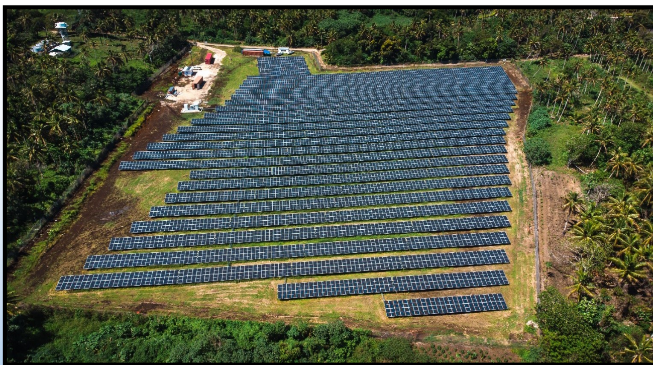
6MW Solar Power Plant in Tonga
