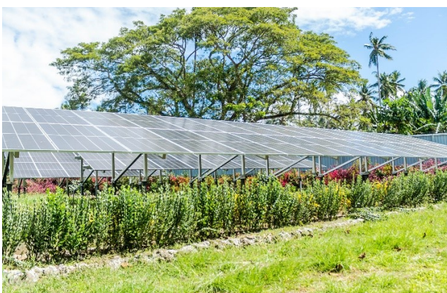
a) PV array at the site
