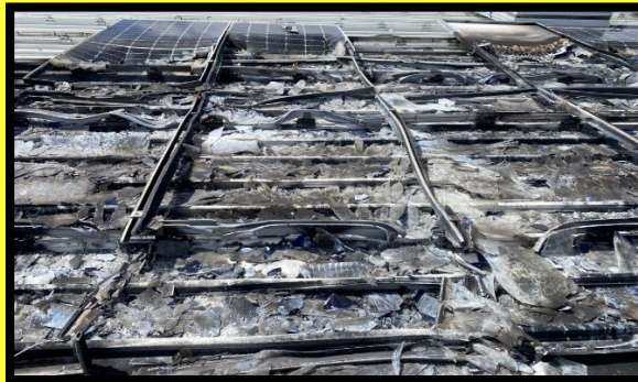
Fire damaged array. Solar fires are headaches for the owner and the installer.
