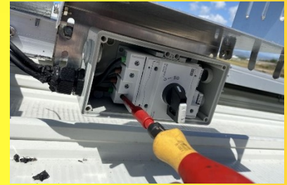
Figure - Torque being checked at a terminal. Always make sure you have tightened all your connections to the manufacturer's specification.
