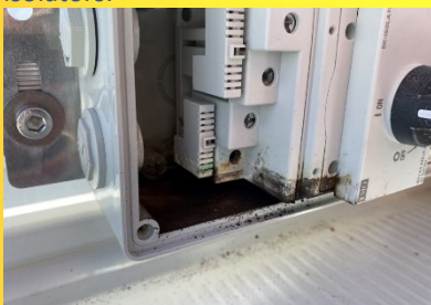
Figure – partial immersion of the isolator and corrosion evident with watermark and presence of green - copper conductor corroded, and brown-iron screw corroded
