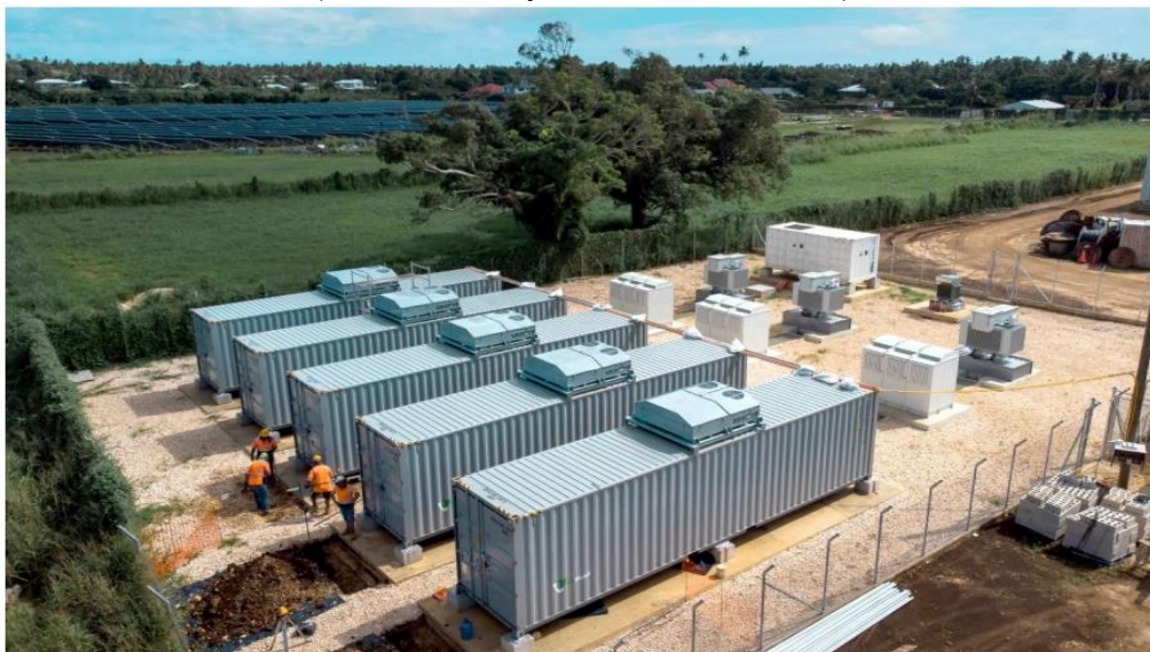
Battery Energy Storage System in Tonga
