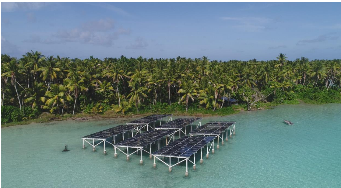
Aerial Photograph of the 77kWp Solar PV Systems at Nukufetau Island
