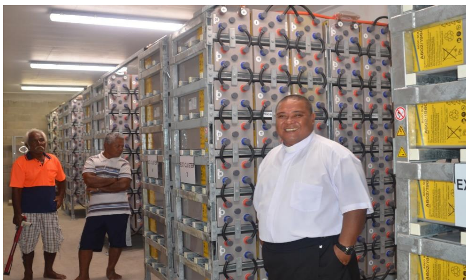
Battery Storage at Outer Islands of Nanumea.
